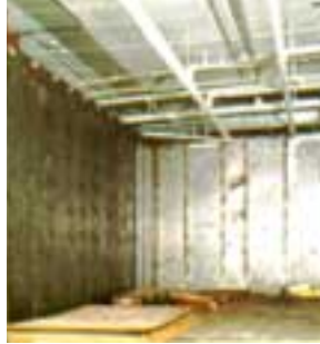
In this second-story, two-vault, Class II installation, the first vault (at left) is complete. Floor and back wall of second vault are under construction.
